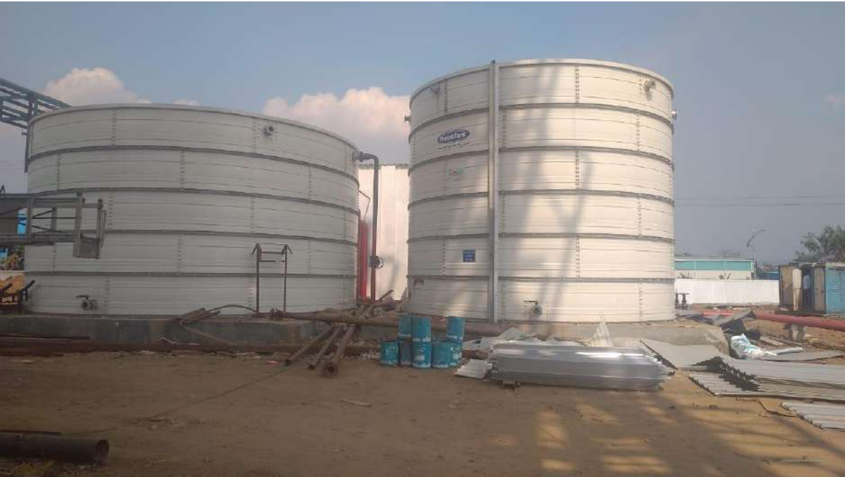
FIRE HYDRANT PUMP STATION
